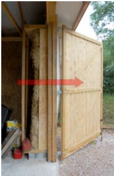
Fig. 5.41: The wall of Paul Douglas' Garage is buckling under compression, perhaps a result of 'bale frenzy'.
