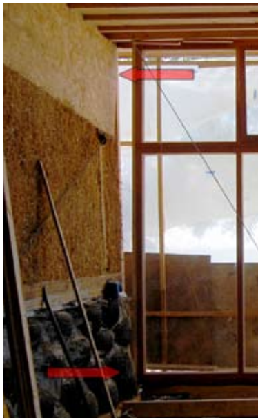
Fig. 5.42: Visible raking in Rik Lander's workshop due to an unforeseen structural issue. The problem is being addressed retrospectively with tensioning cables.
