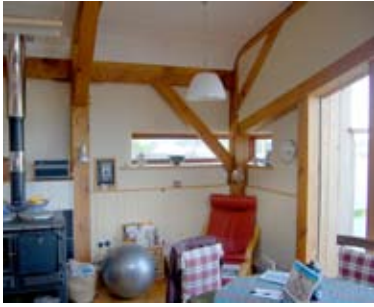
Fig. 3.32: Jim Carfrae's home, an example of straw bale being used as a 'wrap' around a timber post and beam frame.
