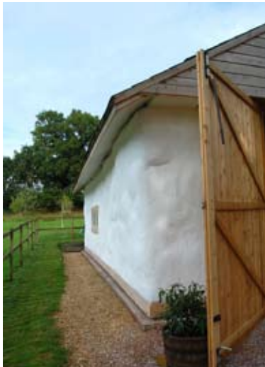
Fig. 4.25: The uneven texture of the finished walls is similar to traditional cob walling.
