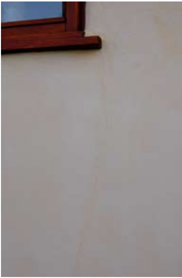
Fig. 5.51: Minor cracks in the render on Carol Atkinson's Straw bale Caravan should be fixed by applying lime-wash.
