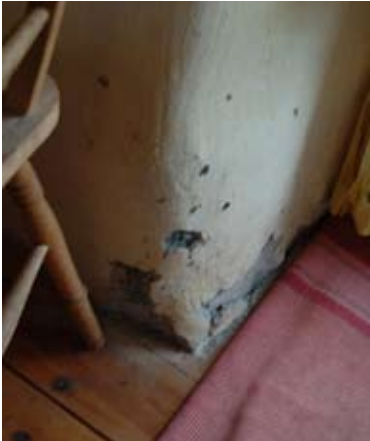
Fig. 5.52: Damage to the bottom of the wall in Kester Wilkinson's Straw House.
