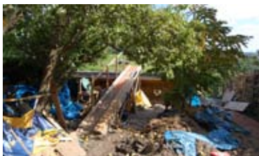
Fig. 4.42: When complete Rik's workshop will blend into the relandscaping of the sloped back garden.
