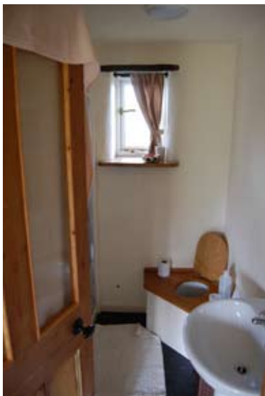
Fig.4.53: The bathroom complete with composting toilet.
