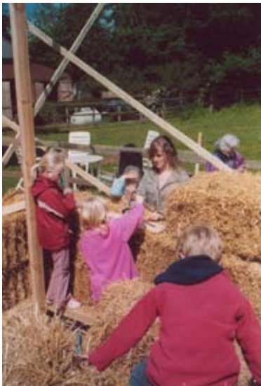
Fig. 3.21: Barbara Jones believes Straw Bale construction helps to involve more people in the building process as demonstrated by children working on Paul Douglas' garage.
