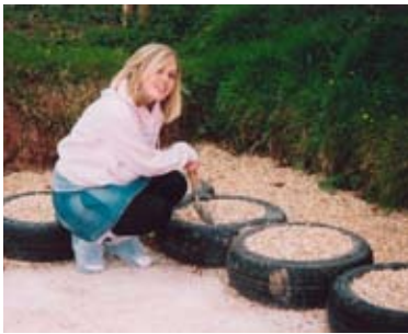
Fig. 5.22: Paul's concrete slab and foundations caused issues with the building regulations officer.
